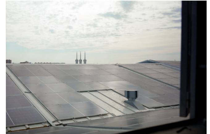
Photovoltaic panels, BioSystems Barcelona.
